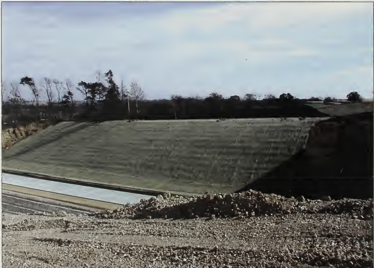
Figure 13 U.S. Highway 151, County A cut circa 2003.
